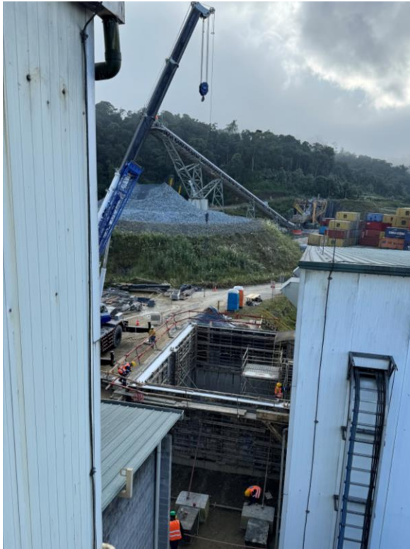
Third concentrate filter building
